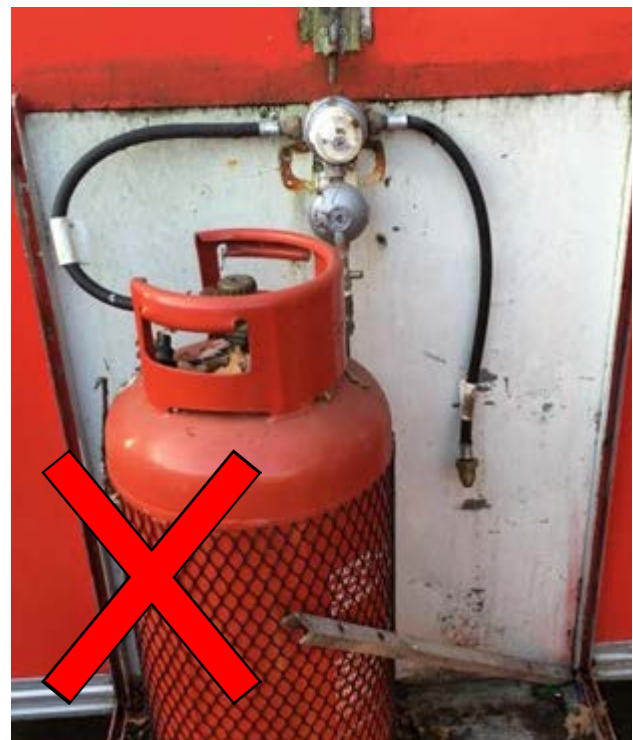
A fixed installation with an unconnected pigtail
