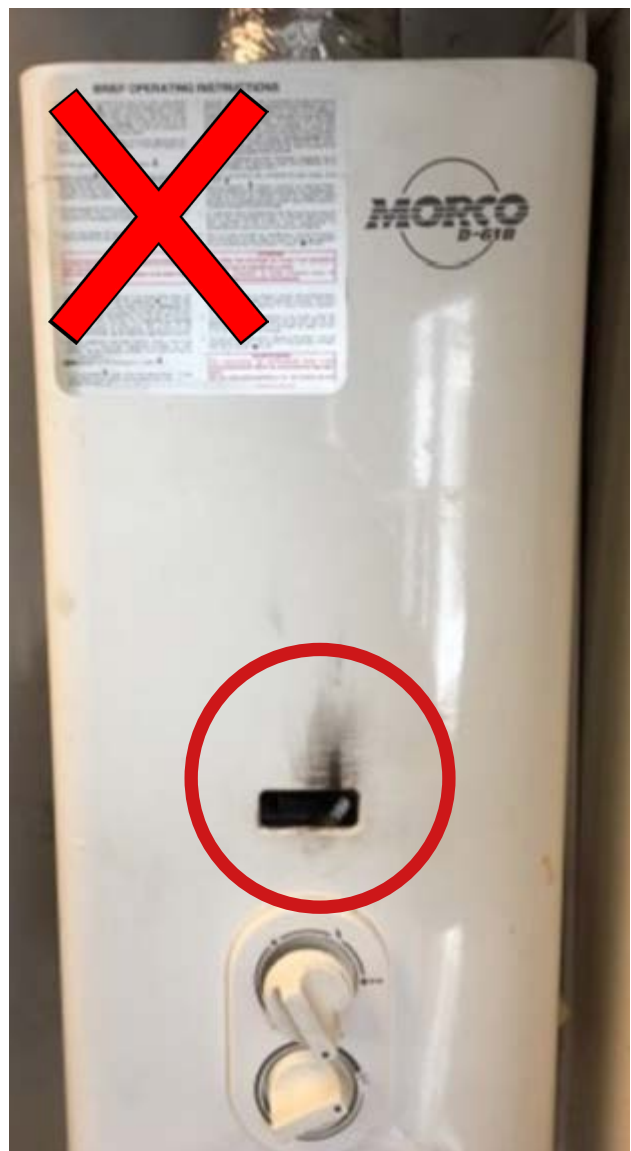
Combustion spillage from a water heater unit in mobile catering premises
