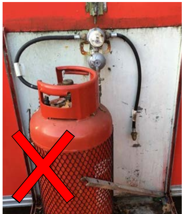
A fixed installation with an unconnected pigtail
